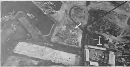
AN ARROW points to the three tank foundations on site at Lago's new Oranjestad bunkering station scheduled for completion Oct. 31. The terminal station will be located between the tanks and the basin in which the small freighter is berthed.
